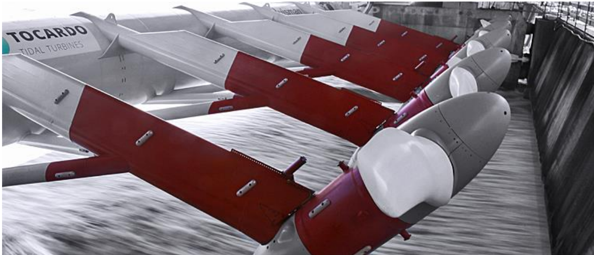
Figure 7: Turbines installed as part of the Eastern Scheldt Tidal Surge Barrier
